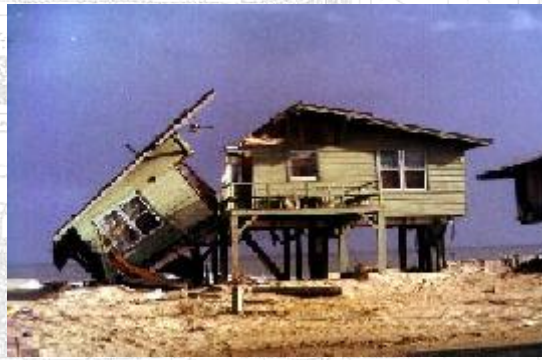
Figure 9: Hurricane Damage, Florida (2004)
